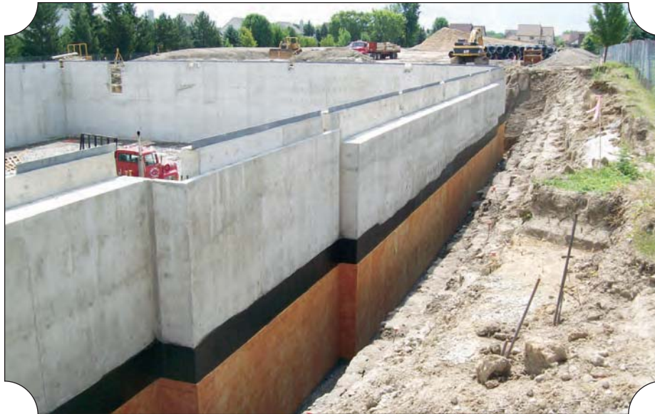
Stante Excavating, Wixom, excavated just over 20,000 cubic yards of soil for the basement. Poured Brick Walls, Inc., Brighton, placed 1,300 cubic yards of concrete and 43 tons of steel reinforcement for the basement.
